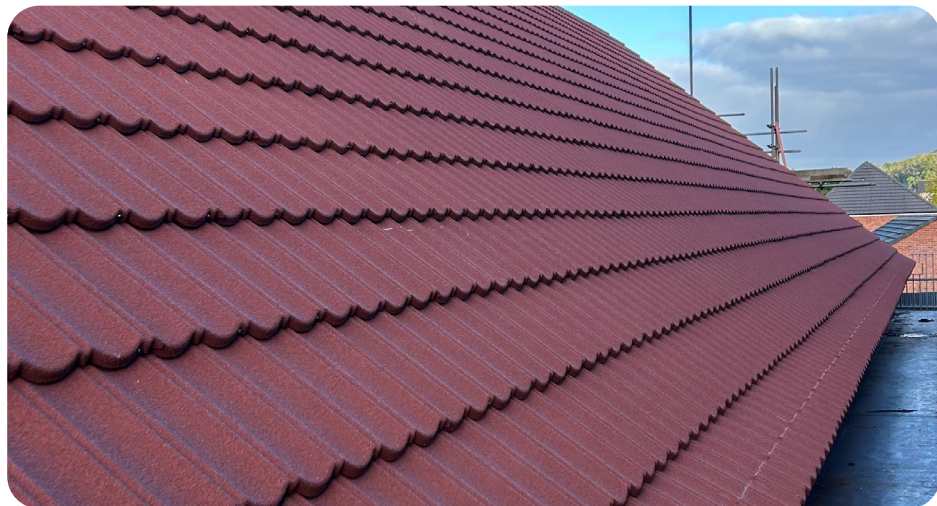
Above: A close up look of the Red Bond .9 tile down the new roof on Immanuel Church.
